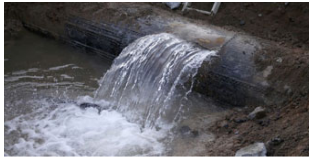
The nation's utilities lose about $2.6 billion annually from leaked drinking water, according to an estimate by the Environmental Protection Agency (EPA).
